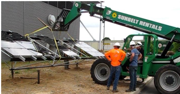
Test installation of 30' QuadPod at Georgia Tech!
