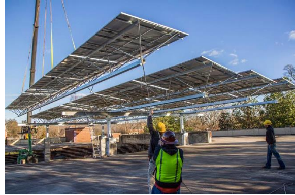
Successful Completion of Agnes Scott College pilot project installation: (Taken: 12/16/14 )
