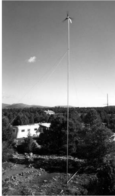
A Southwest Windpower Air 303, 300-watt turbine is the sole source of electricity for this remote home in northern Arizona.
