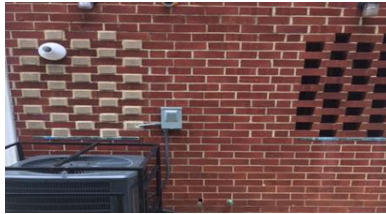
Townhome (left) with AC upgrade and venting for a high efficiency furnace (white pipe above AC unit) next to a home (right) that did not income qualify and still has natural ventilation holes in the wall for a low efficiency furnace. Note the concrete slabs for AC condensers were contributed by the landlord.
